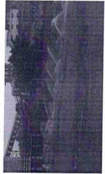
Fixed type dust suppression system
