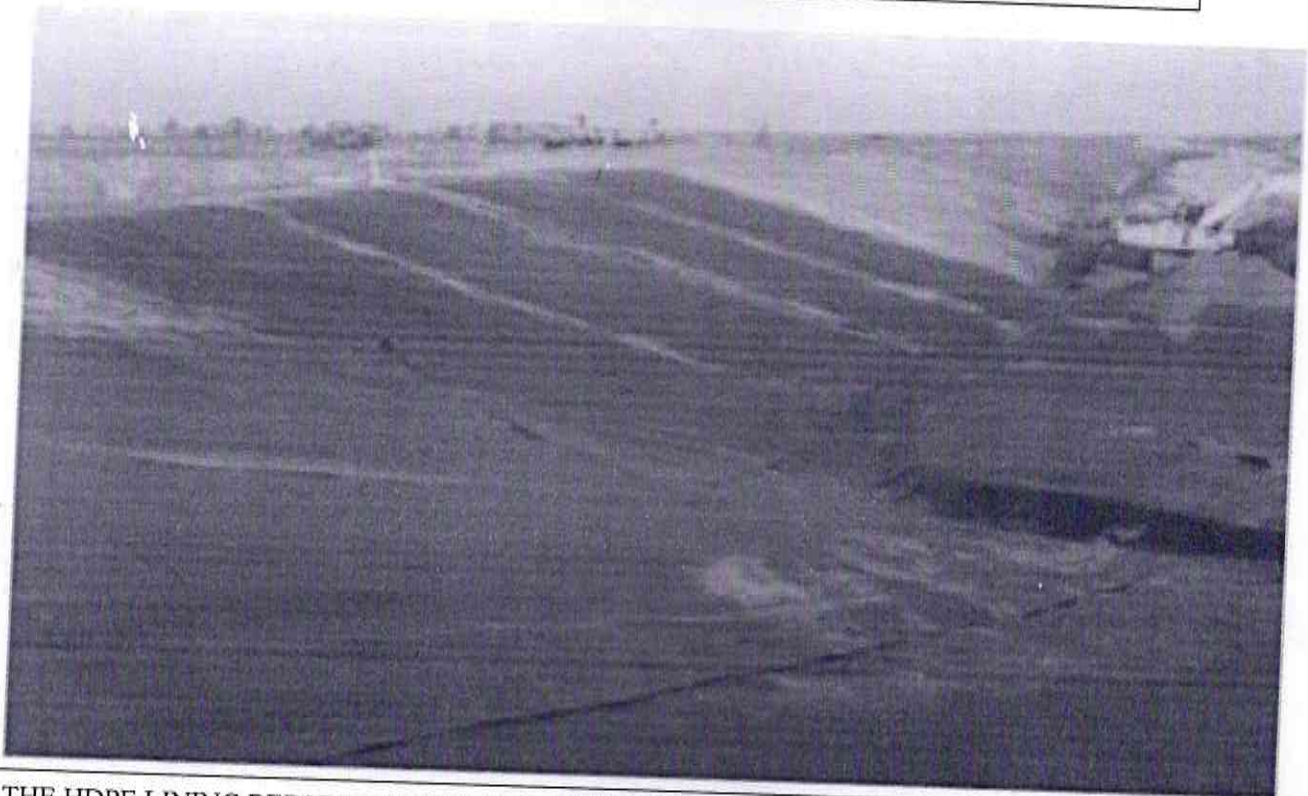
THE HDPE LINING BEING PUT OVER THE BOTTOM BED OF ASH POND NO. - 2 (PHOTOGRAPH - 10)
