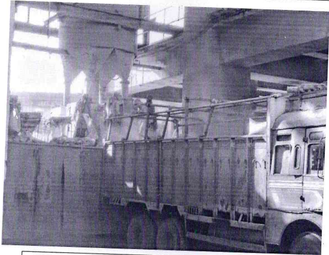
SILO ASH BAGING READY FOR DISPOSAL (PHOTOGRAPH-15)
